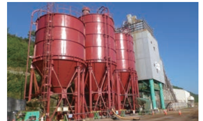
Dedicated "ash-crete" plant.
