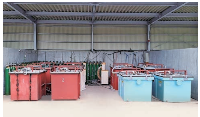
Granulated recycled aggregate carbonizing equipment.
