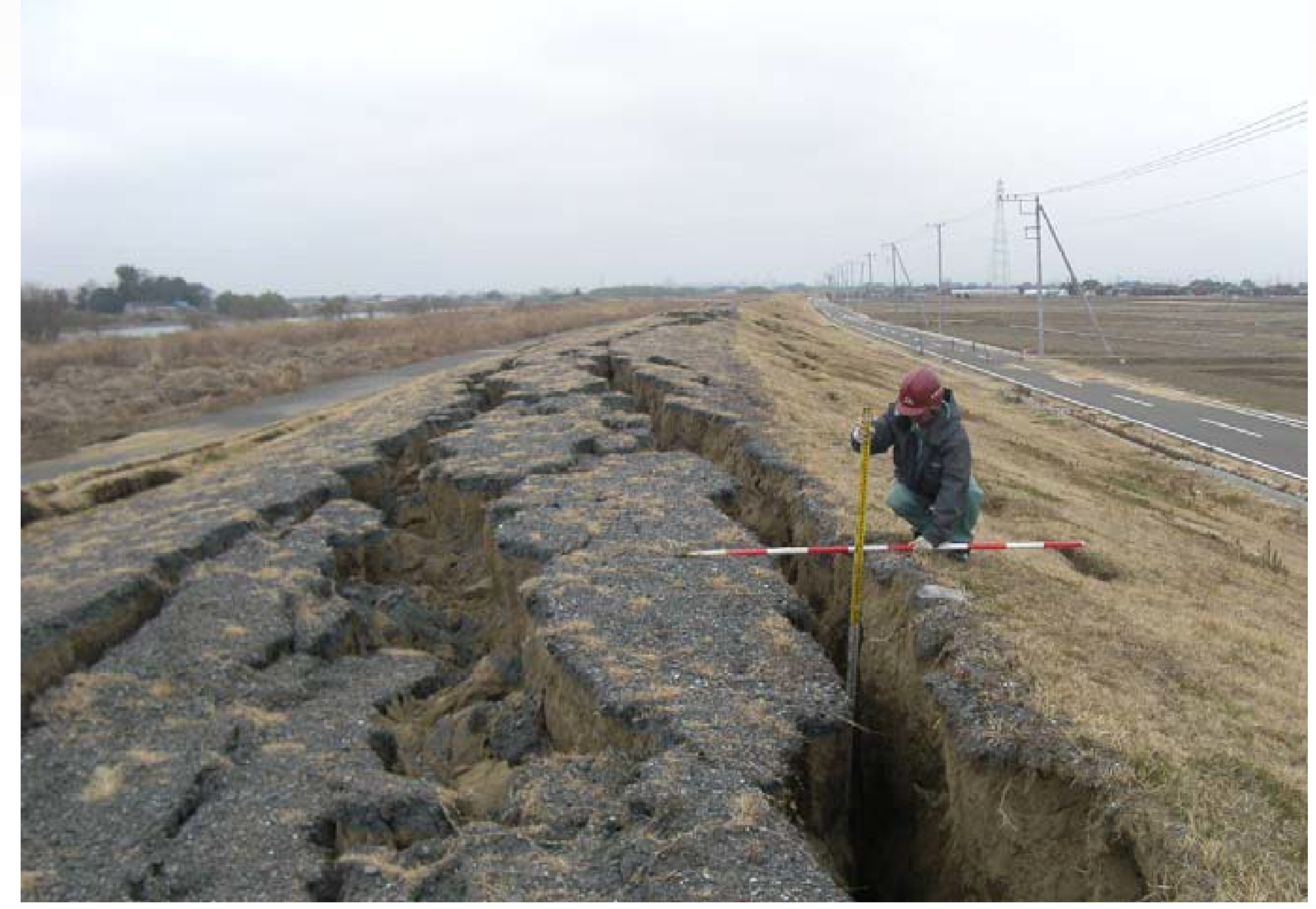
Earthquake Damage to Riverbank (Naka river, Ibaraki Pref.)
