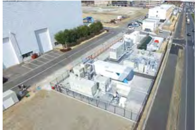
Next-generation low-CO 2 cogeneration plant
